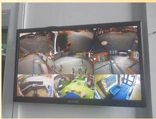
CCTV System at Kingsfield First
